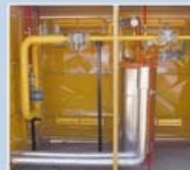
IRS / Evaporating regulating station
