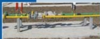
Pretakalni most / Charging equipment
