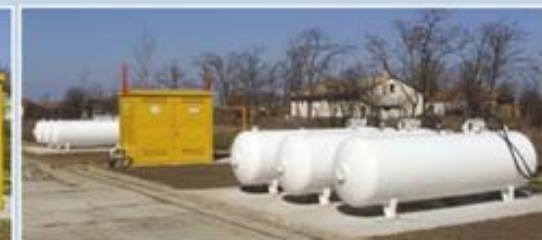
Postrojenje propan-butan gasa / Liquid petroleum gas facility
